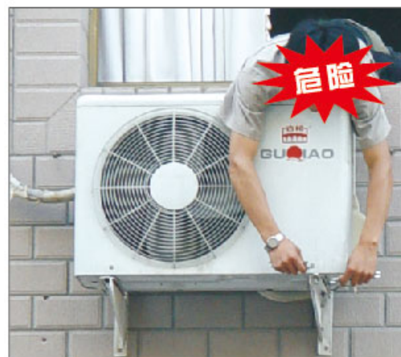
Very dangerous 非常危险
